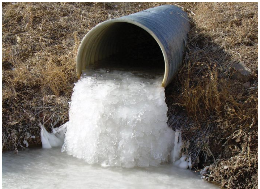
The effects of freezing in a culvert.
