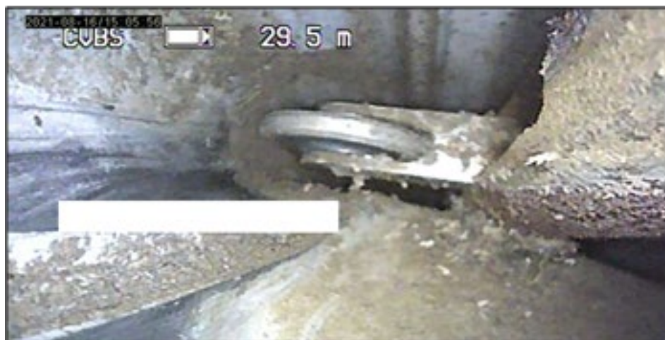
Figure 4: Aluminum inclinometer casing obstruction, Dam 1 Section A
